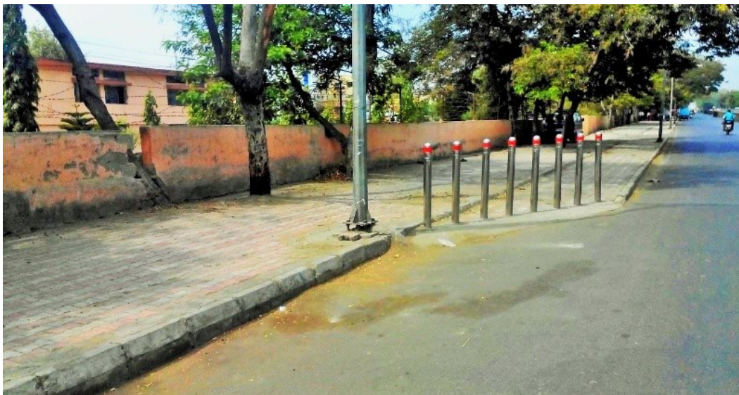
Figure 8: Ill designed cycle lane with bollards breaking the continuity
