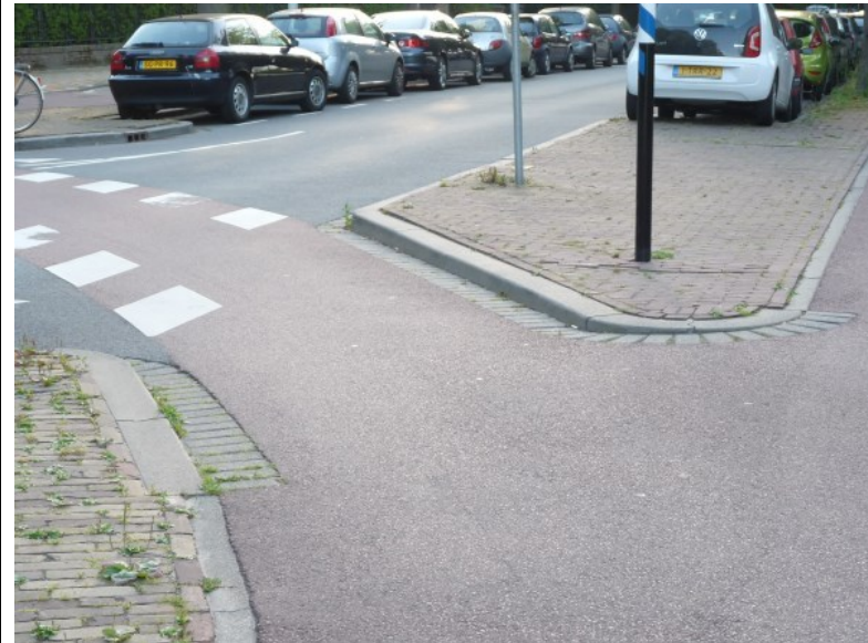
Figure 43: A smooth road surface, also at intersections, leads to better comfort.
